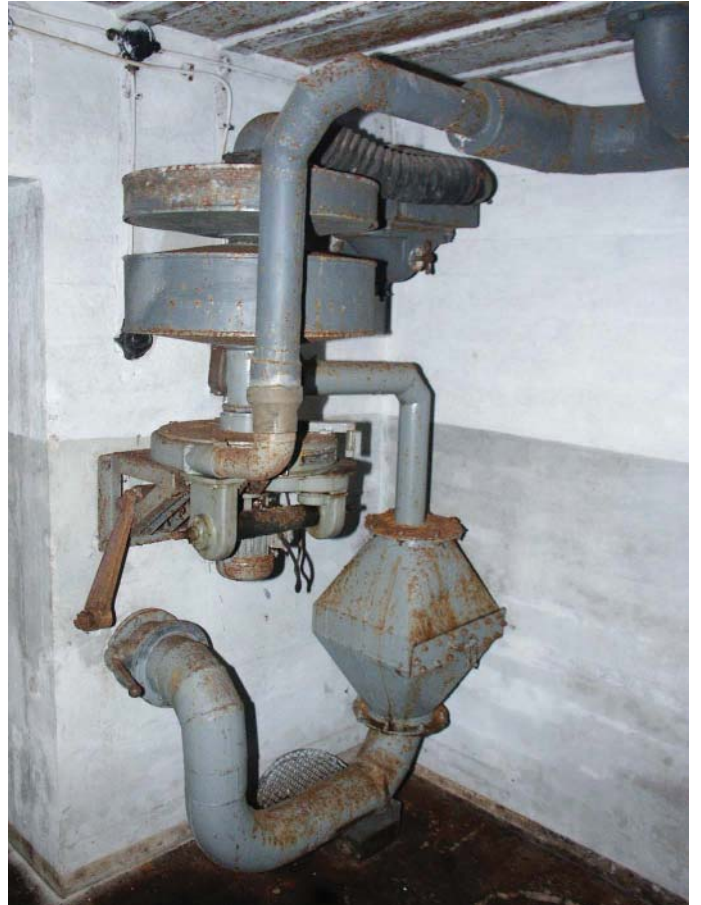
Lista Vestre Hauge: main air-filter called HES 2,4 ( one new filter added postwar ),
